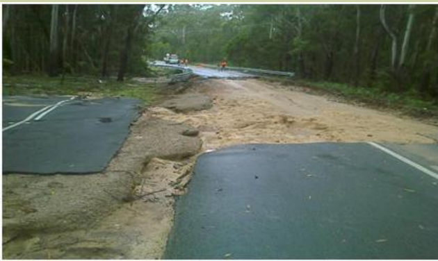
A section of road at Diana's Basin near St Helens which was washed away in January 2011. Reedy Creek Bridge is in the background.
