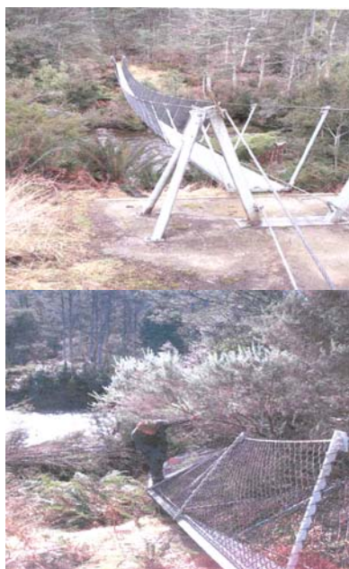
The Pine Hut Plain, Mersey River suspension bridge, before and after the storm
